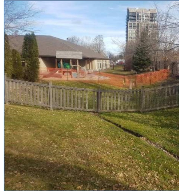
Figure 20: The second surface drainage feature downstream of the end of the culverts, south of the River Parkway Childcare Centre's playground; photo taken November 12, 2020.
