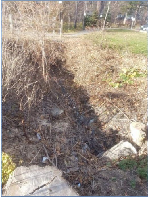
Figure 10: Upstream portion of the first surface drainage feature, at south central part of the property, coming from between the parking lots on the Old Rail Line area; photo taken November 12, 2020.
