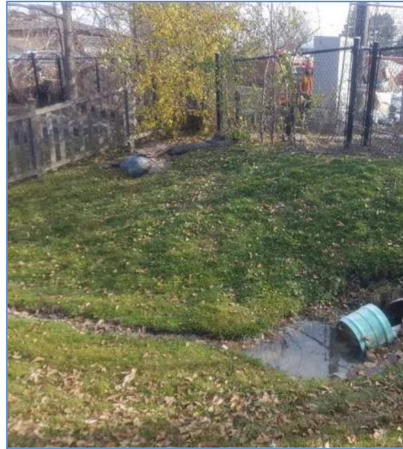
Figure 19: Downstream end of culvert and source of the second surface drainage feature, at southwest corner of the River Parkway Childcare Centre's playground; photo taken November 12, 2020.
