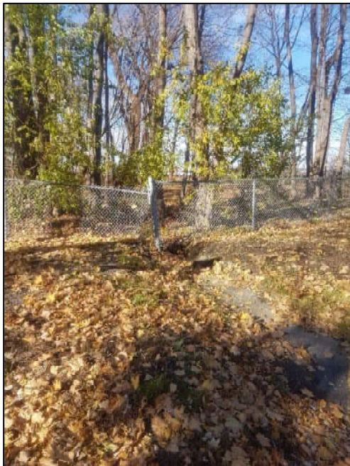
Figure 79: Paved drainage feature, for conveying stormwater from parking lot; photo taken November 12, 2020.
